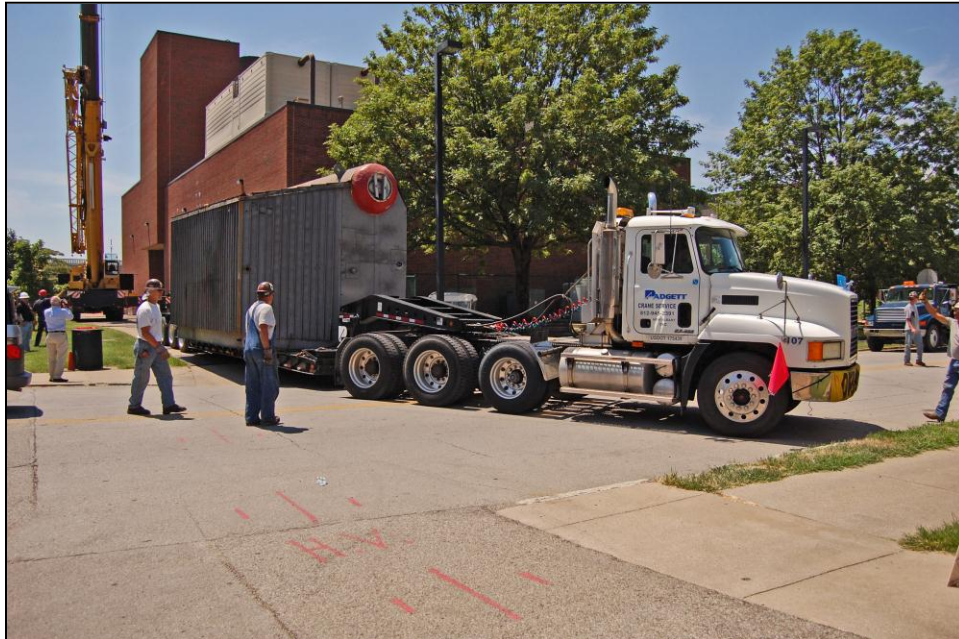
UofL sends its old coal-fired boiler to the recycler, replacing it with a cleaner natural gas boiler in the summer of 2010.
