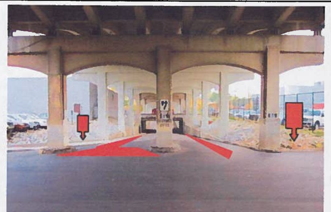
Old Eastern Parkway with bike lane markings and way-finding signs; connects to Brook.
