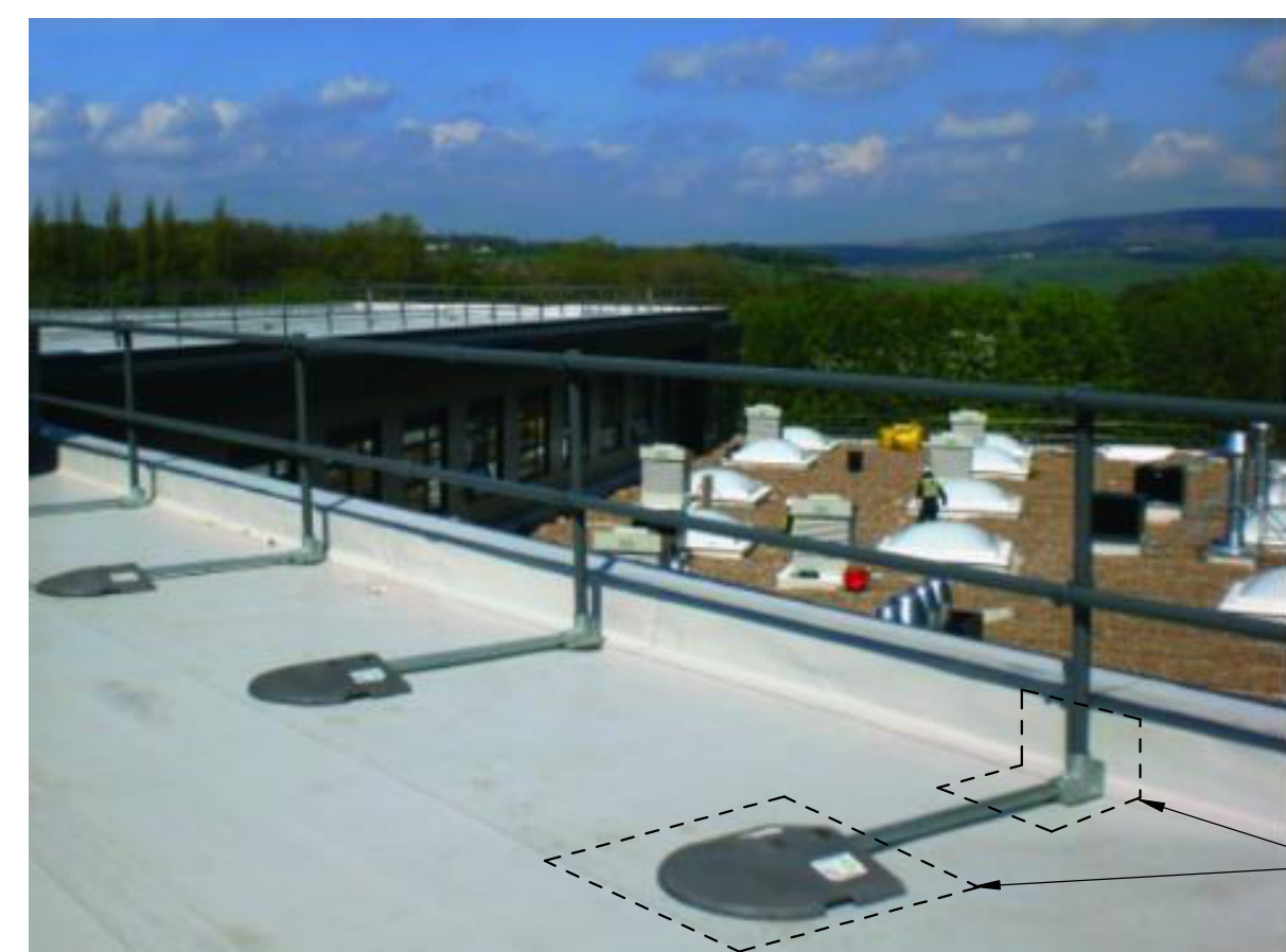
PROVIDE ROOF PROTECTION PADS AT EACH BEARING POINT. ADHERE PADS TO ROOF.
