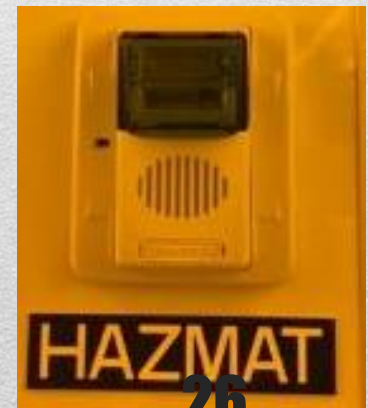
Hazmat Alarm (Blue Strobe)
