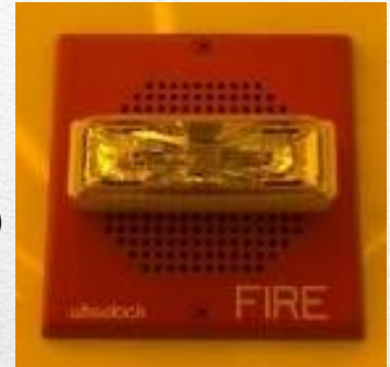
Fire Alarm (white strobe)
