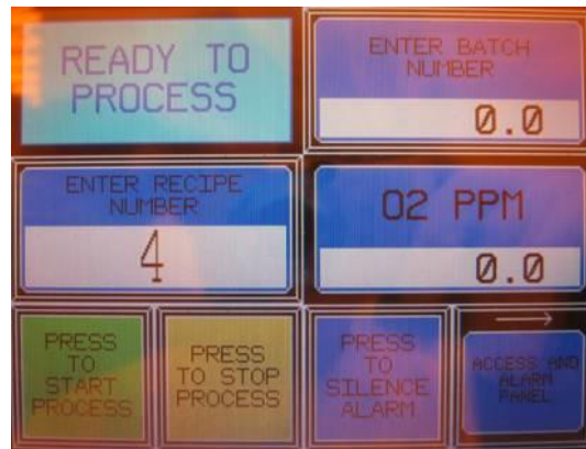
Operator's Touch Screen Panel
