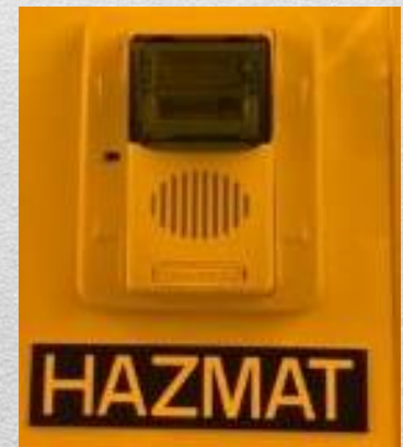
Hazmat Alarm (Blue Strobe)
