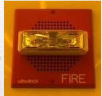
Fire Alarm (white strobe)
