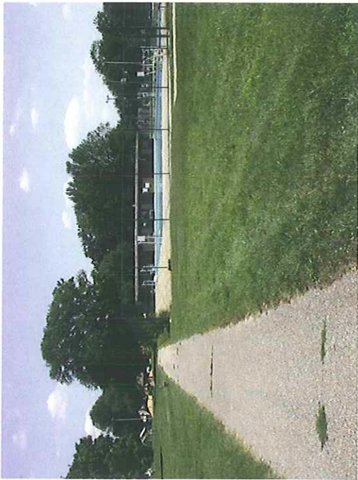
Existing pool to be renovated. Pedestrian path to be redesigned and replaced.
