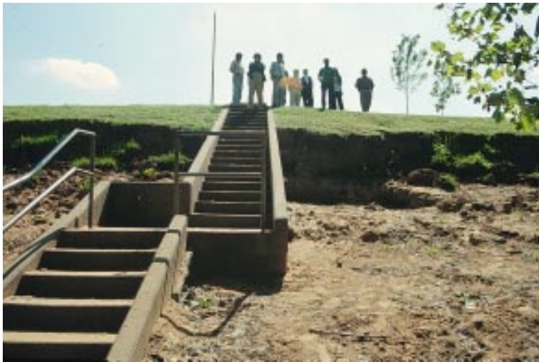
Bank erosion at Riverview Park.
