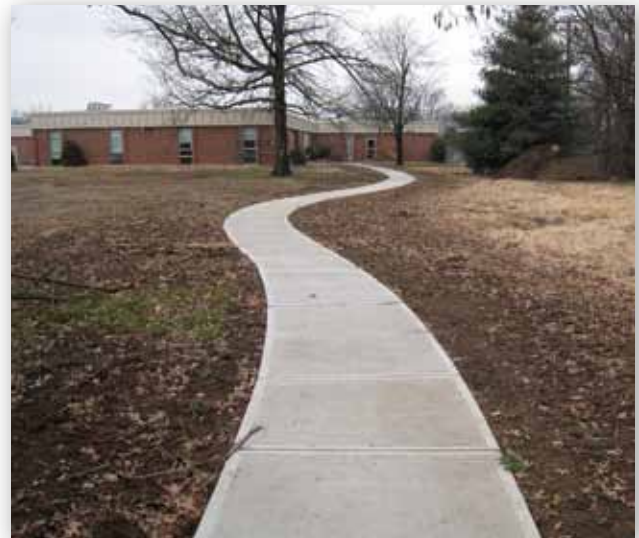
A newly-installed concrete pathway loop at Cane Run Elementary School provides complete access for all students to the numerous planned learning zones around the approximately 10-acre schoolyard
