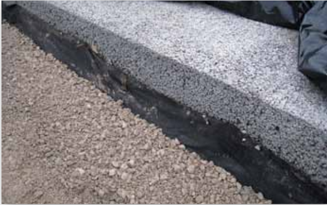
Permeable concrete surface being installed at Cane Run Elementary School in Louisville, Kentucky
