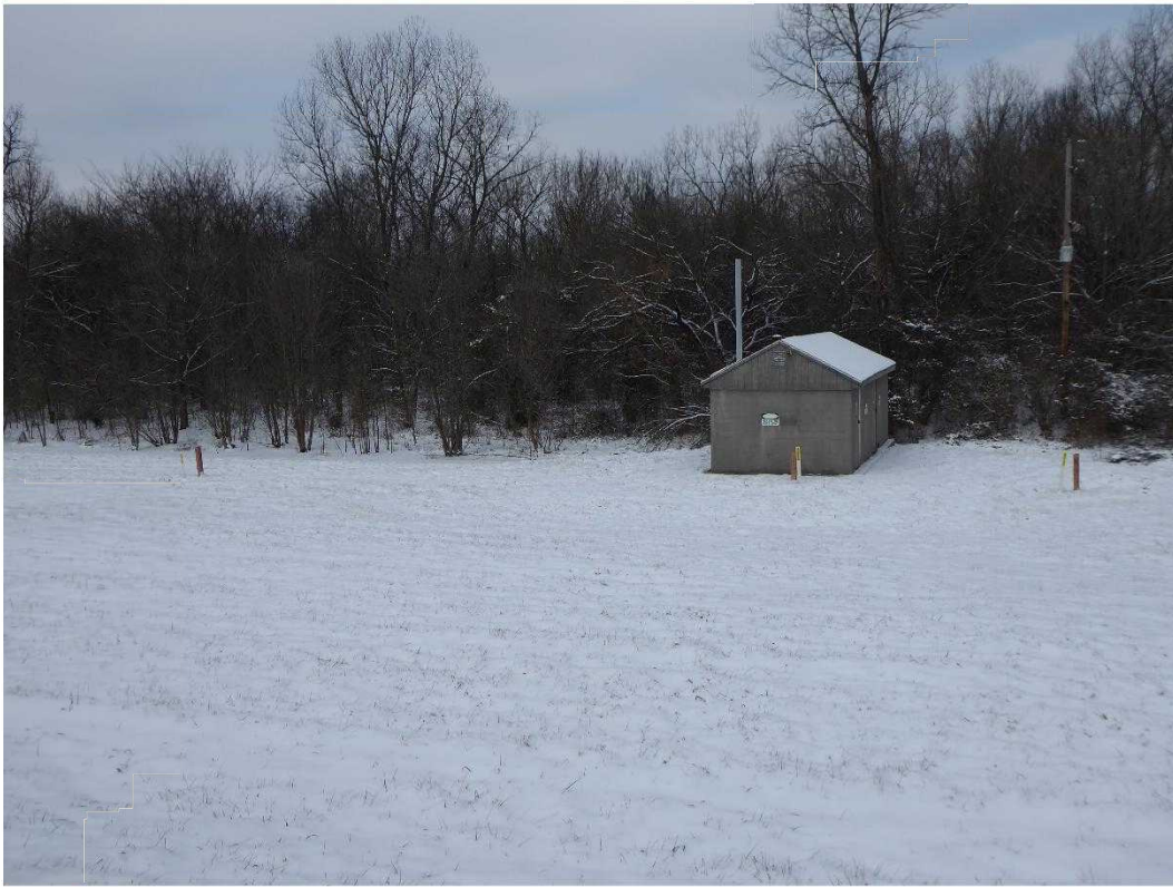
Blower house for gas extraction system near Lee's Lane, on northeast corner of the Central Tract
