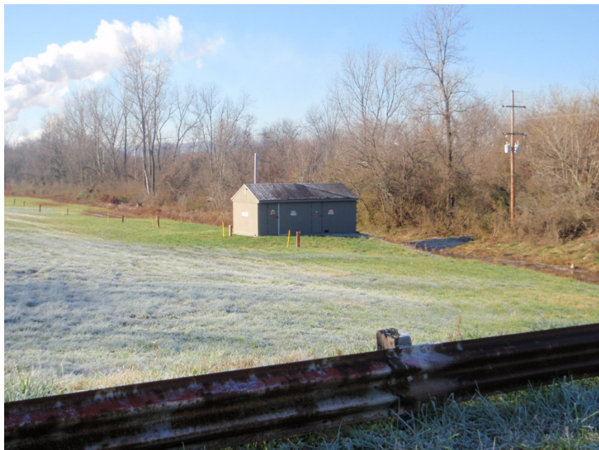
Wells along the gas extraction system and the blower house for the gas extraction system.
