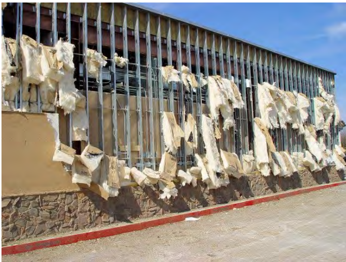
The 2008 tornadoes impacted critical community infrastructure and facilities across the state, like this hospital in the city of Mountain View, in north central Arkansas. Credit: Vaughan Wingfield, UALR Institute for Economic Advancement.
