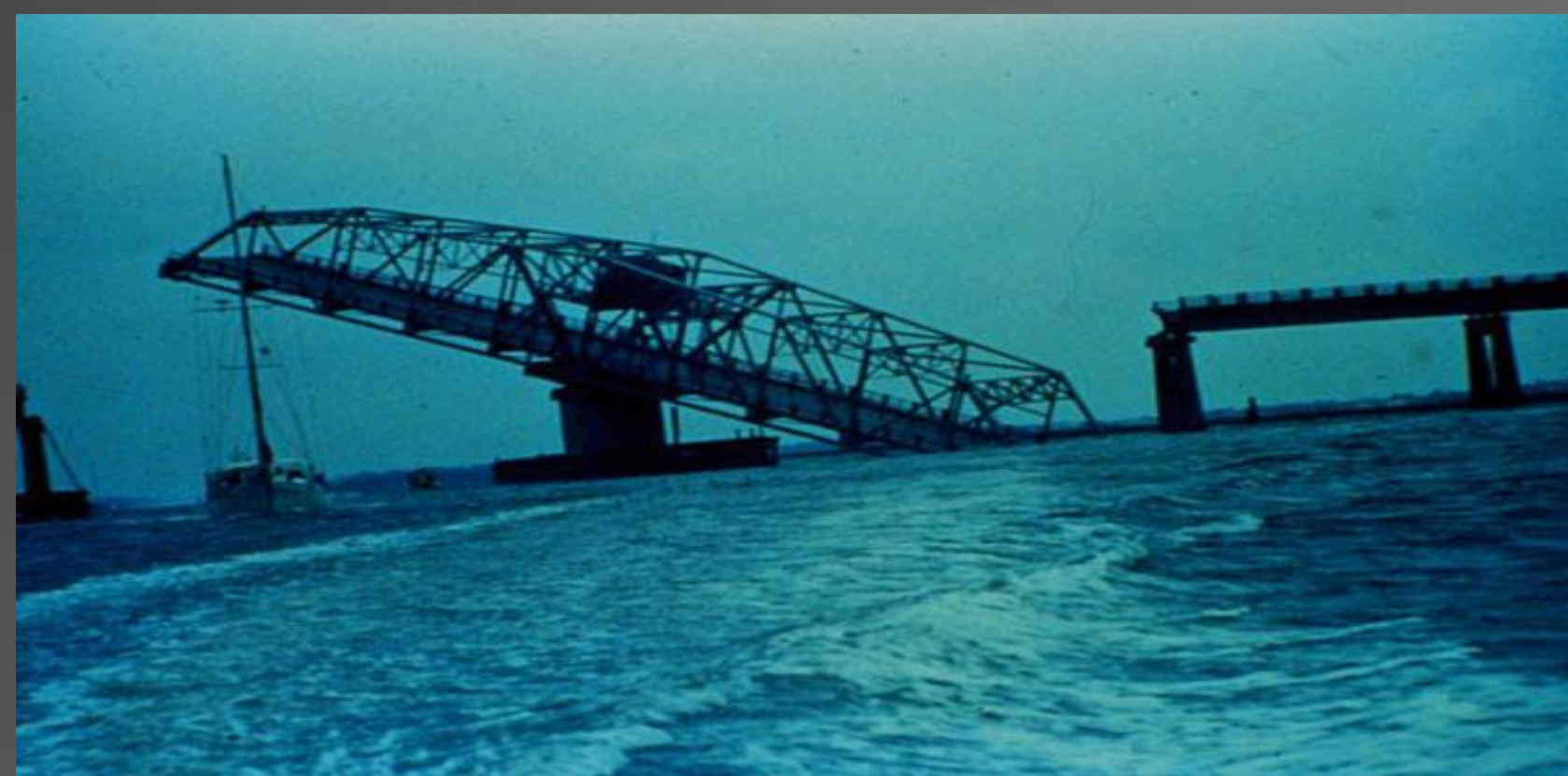
The Ben Sawyer Bridge to Sullivan's Island, SC sags into the water. NOAA.
