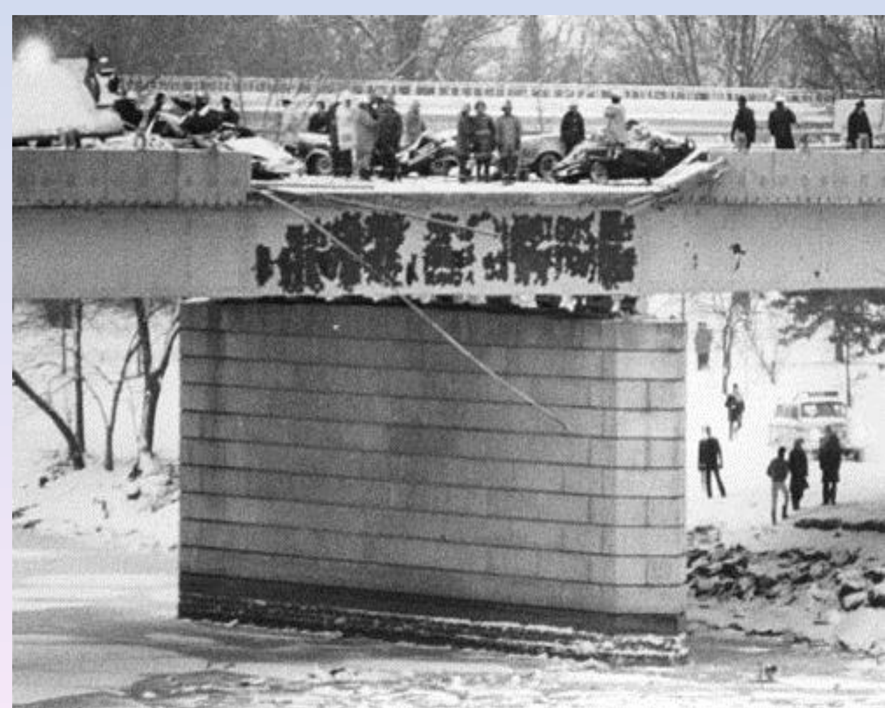
Photograph showing the section of the 14 th Street Bridge damaged by the crash. Photograph courtesy of The Washington Post .
