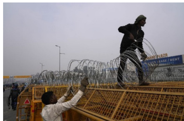
Workers constructing barricade to prevent protestors from entering New Delhi. Source: AP Photo/Manish Swarup
