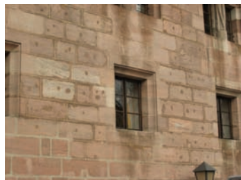
Bullet holes in the side of a building.
