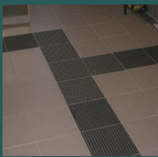
The facilities at START were very handicap friendly. One special feature was this tiling on the floor which assists blind individuals with navigating the hallways. Tiles are ridged with bumpy tiles places at
