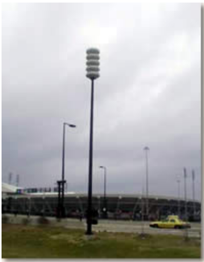
Outdoor Warning Siren at Papa Johns Cardinal Stadium.
