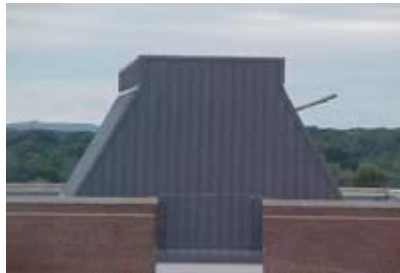
Notice the tree branch that penetrated this sheet metal wall. (University of Maryland)
